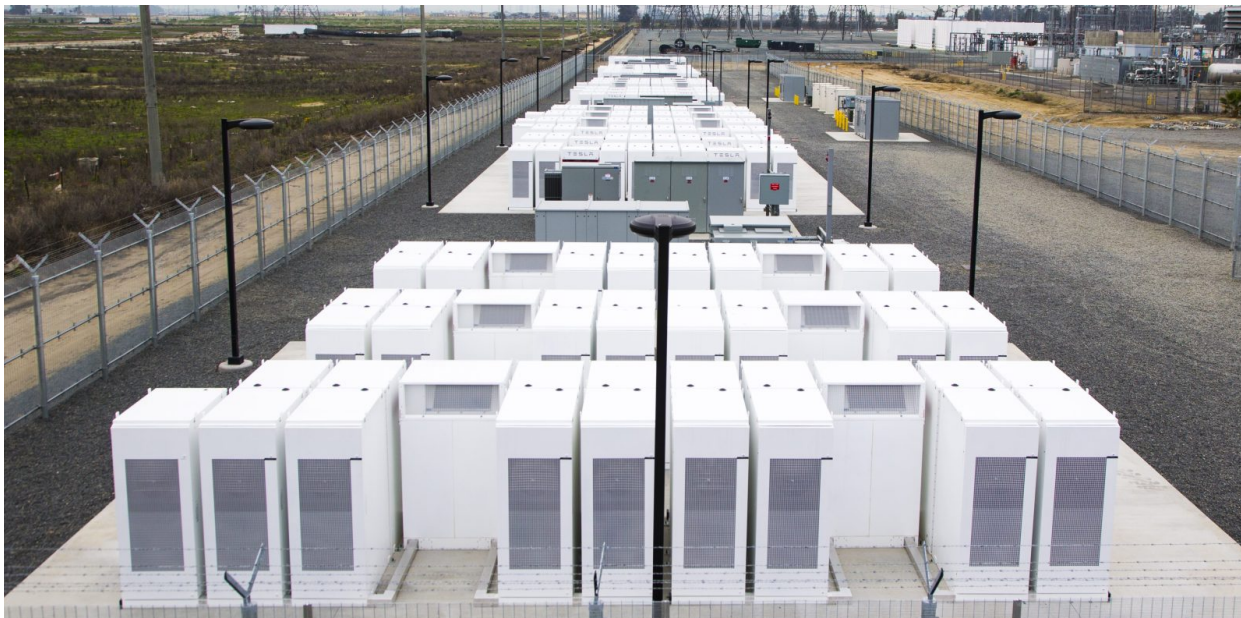
Figure 9: 20 MW battery system with 4-hour storage capacity (80 MWh)
