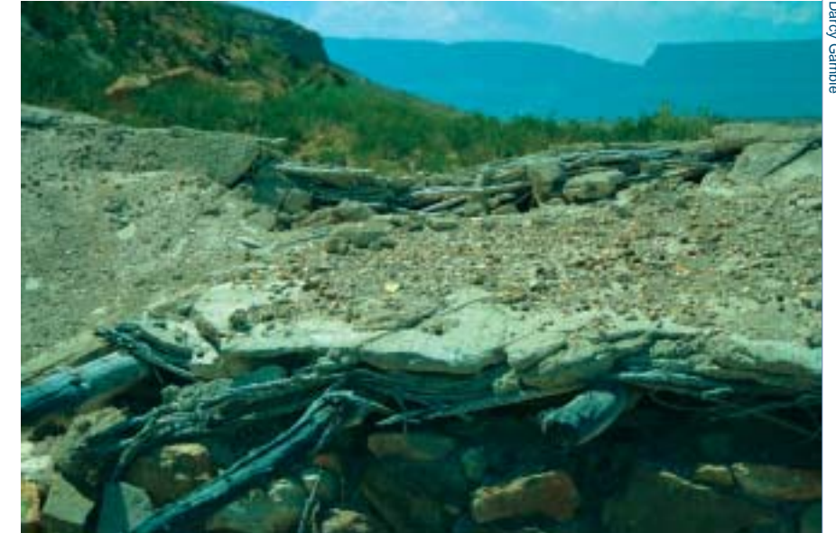
Luna's Jacal, an earthen abode built in the 19th century, is listed in the National Register of Historic Places. The park has been unable to repair the roof of this nationally significant structure because of lack of funds.
