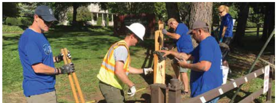
Above: Veterans with The Mission Continues line up a new fence at Fort Vancouver National Historic Site on September 11, 2016. ©Rob Smith | NPCA
