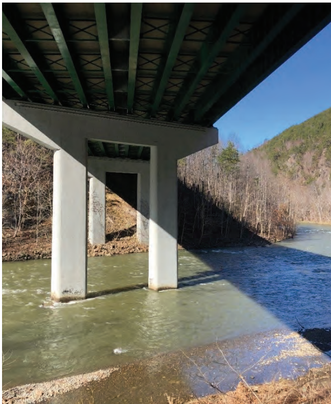
Pigeon River Bridge in Tennessee. Photo: Wildlands Network
