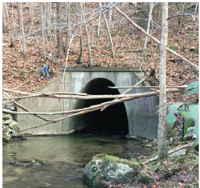
Hurricane Creek Culvert. Photo: NPCA
