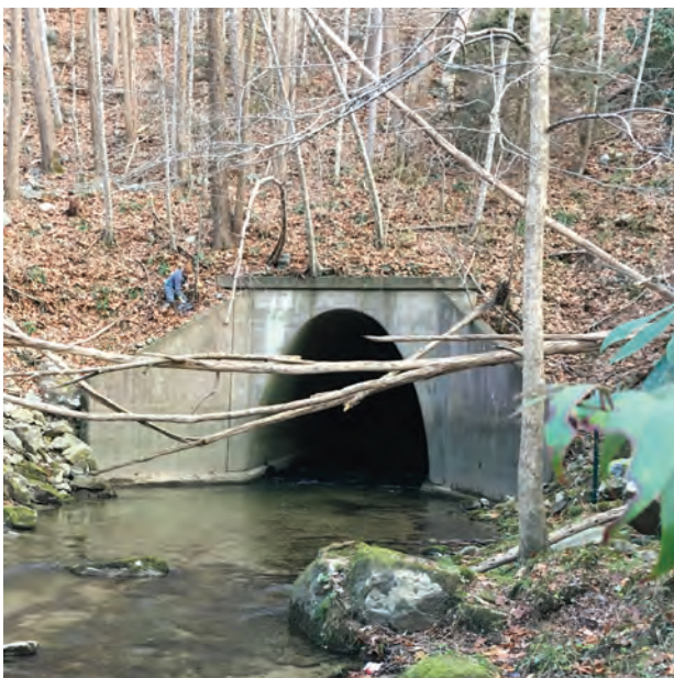
Hurricane Creek Culvert. Photo: NPCA
